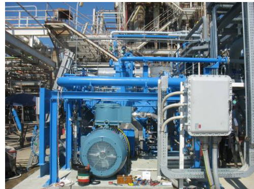
Figure 21: Compressor controlled by VSD
