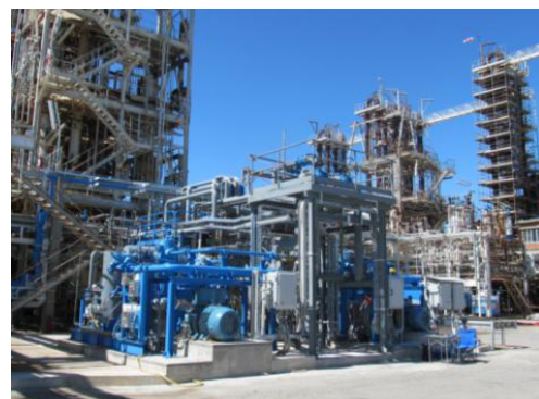
Figure 15: New compression and interstage condensing plant after the revamp of August 2013
