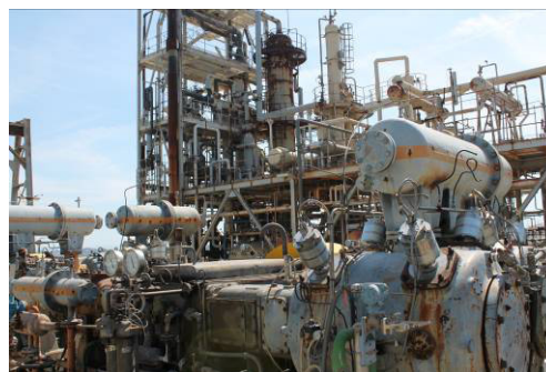
Figure 7: Compressor with the installed capacity control system
