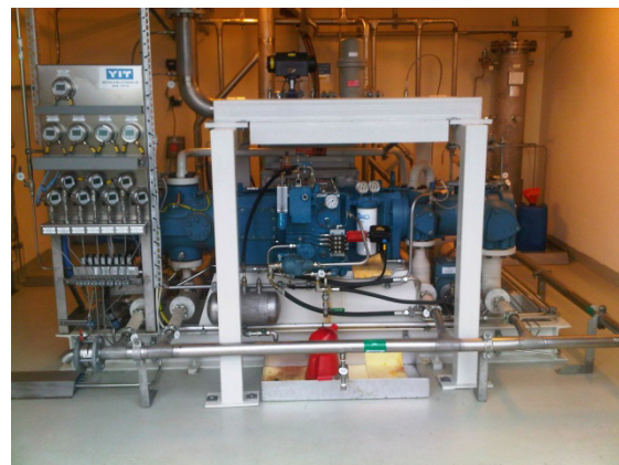
Figure 2: One of the three natural gas compressors at the Helsingborg bus station.
