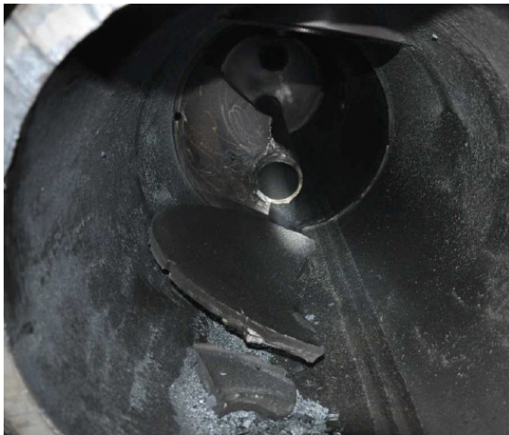
Figure 5 Failure of the baffle plate of the discharge 1 st stage damper (outlet side)
