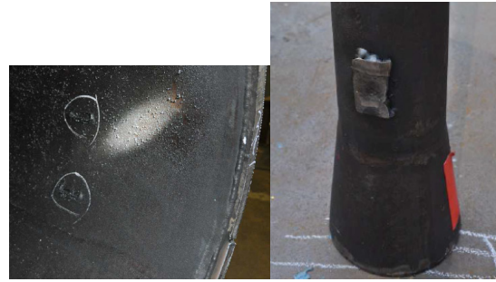
Figure 7 Broken brace of the baffle choke tube of the discharge 1 st stage damper (inlet side)
