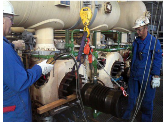
Figure 5: Source HTC Zero-leakage sealing system installed on a compressor at Den Helder.
