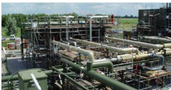
Figure 1: source NAM The Den Helder gas treatment plant
