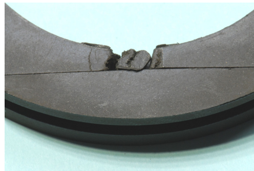
Figure 2: Failure by fracture near the joint of a packing ring with limited wear
