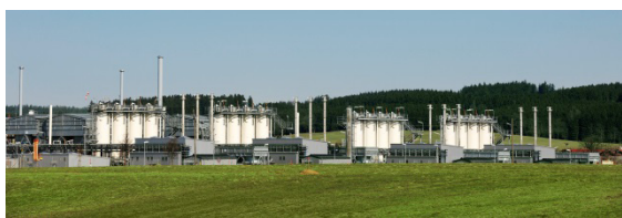
Figure 1: Overview of the Haidach storage facilities (UGS Haidach)
