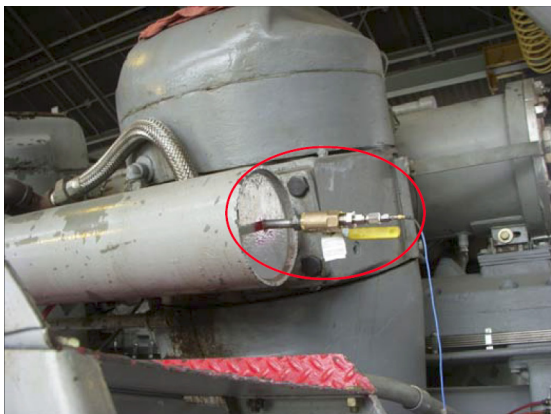
Figure 6. Pressure Transducer Installed at End of Manifold – Test Point P5
