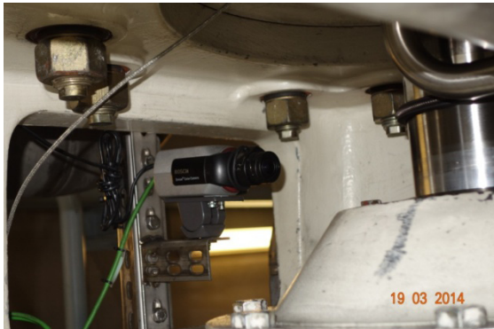
Figure 11: Camera Installation for Continuous Piston Rod Observation Concerning Oil Film Development
