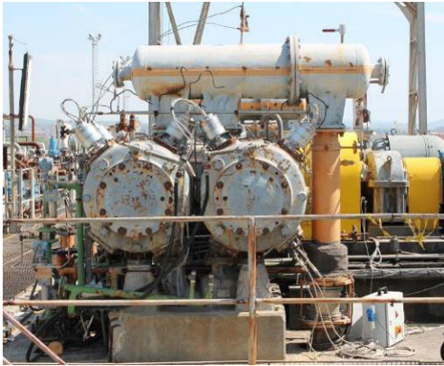
Figure 8: Compressor with the Cozzani portable acquisition system installed
