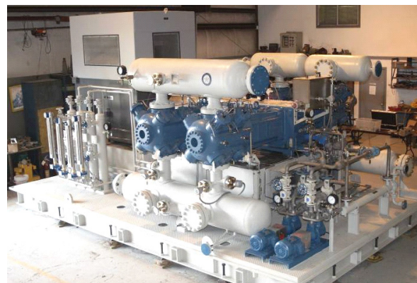
Figure 5: Reciprocating compressor package 4
