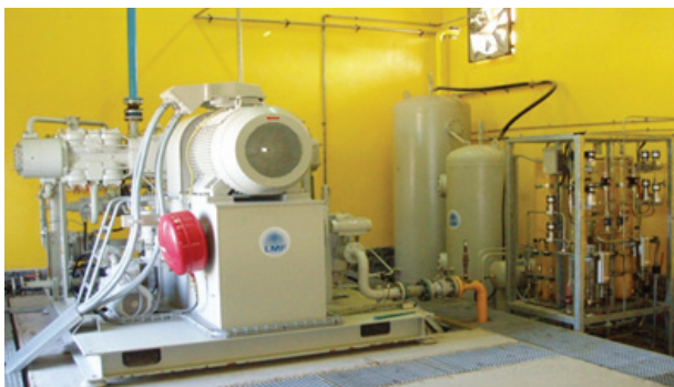
Figure. 4.2.1: natural gas compressor station
